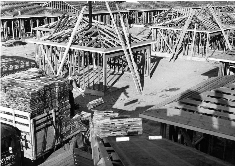
FIGURE 3. Lakewood under construction. Mass production, using assembly line methods and specially designed power equipment for replicated tasks by division-of-labor crews—this was truly a “housing machine.” Both images courtesy of the City of Lakewood’s collection.
